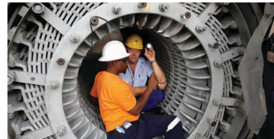
Marthinusen & Coutts divisional CEO Richard Botton and senior artisan Shepherd Chigwa inspecting the 60 MW generator stator at Kelvin Power Station prior to repair.
