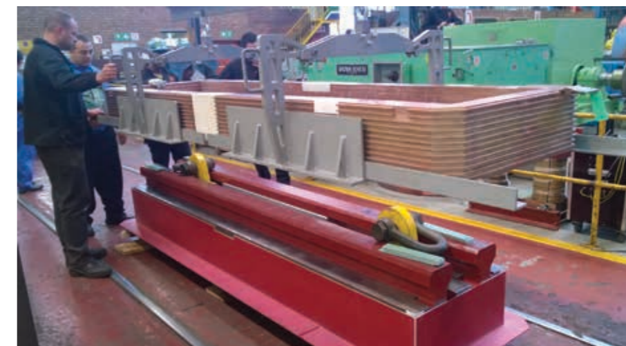
Andrew Step, final year apprentice fitter and turner and qualified armature winder, Ricardo Bernardes, lower a refurbished field coil for Ingula onto its pole body using a custom rigging tool that applies even pressure along the coil surface.
