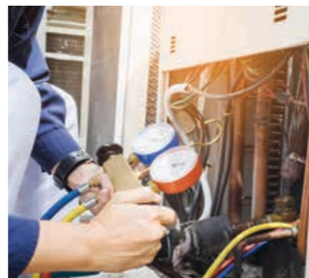
For safe HVAC installations, modifications, maintenance and repairs, only registered SAQCC Gas practitioners should be used and a Certificate of Conformity received.
