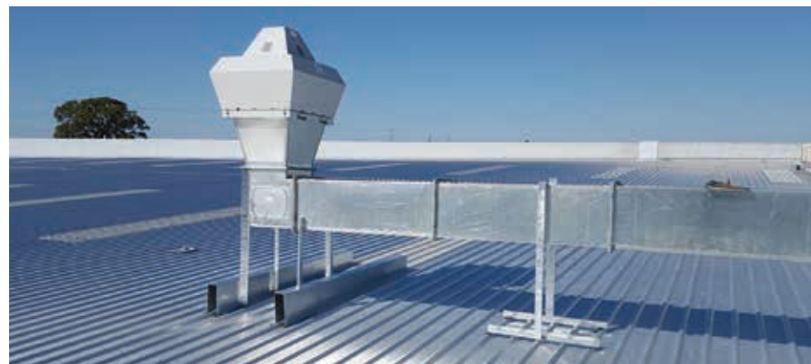
HVAC systems are a big investment. This fact often comes to light when an entire air conditioning system must be replaced due to poor maintenance.
